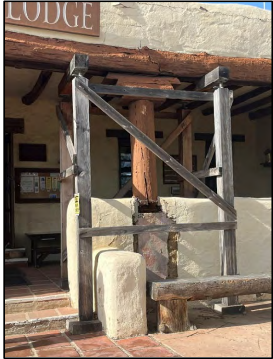
Lodge entryway column scheduled for repair
