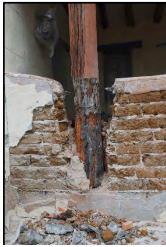
Outer left column showing significant rot and previous alterations
